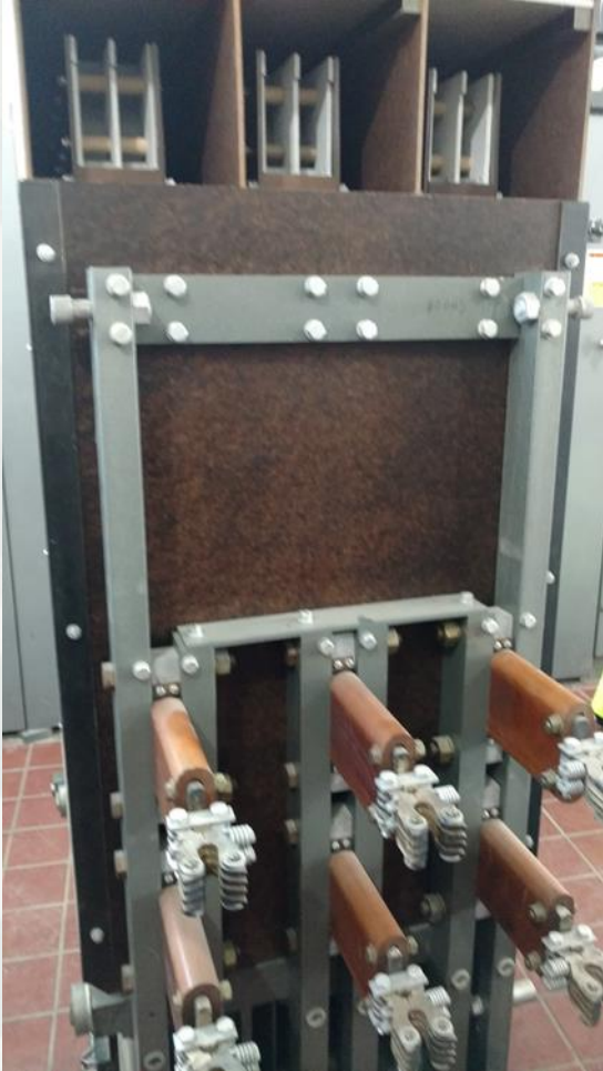
1948-vintage 480V electrical breaker at McNary
